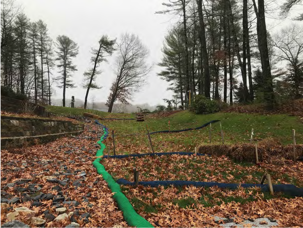
Fig 3: Slope above the manhole at Gundalow Landing/east side of the bay. Viewing east. (12-01-20)
