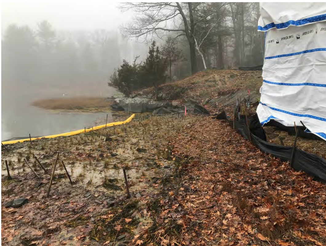
Fig 2: Toe of the slope and salt marsh restoration at the Eversource property/west side of the bay. Viewing south. (12-01-20)
