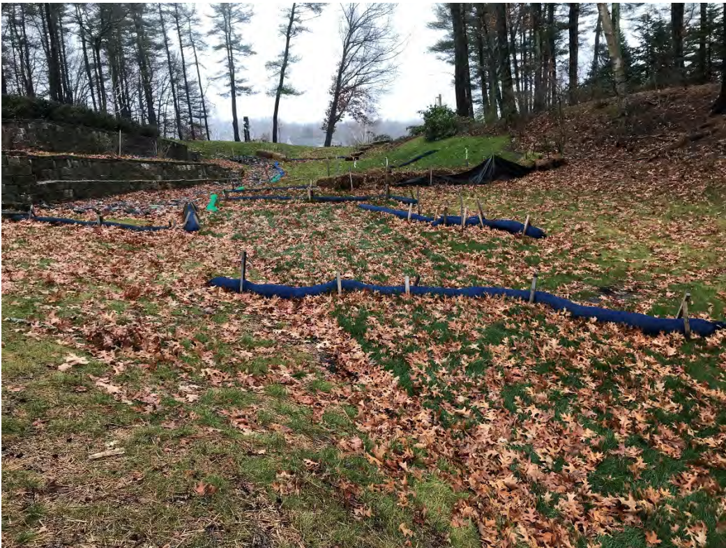
Fig 4: Slope below the manhole at Gundalow Landing/east side of the bay. Viewing east. (12-01-20)
