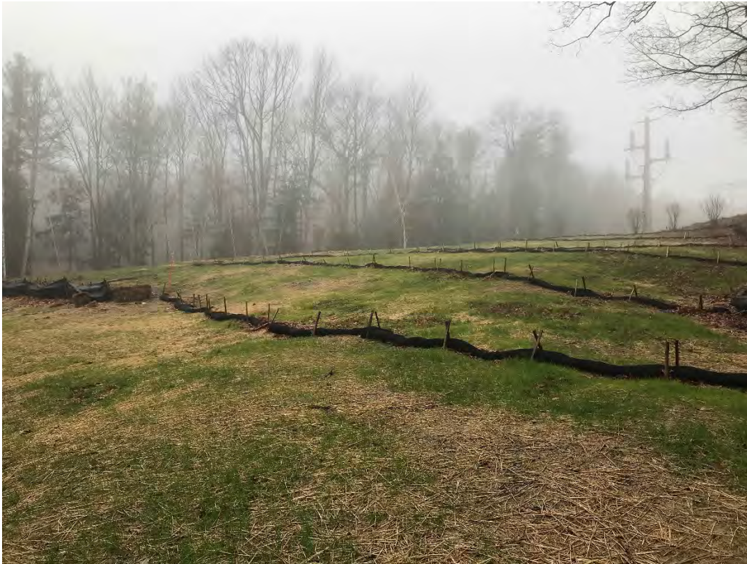
Fig 1: Slope above the cable house at the Eversource property/west side of the bay. Viewing southwest. (12-01-20)
